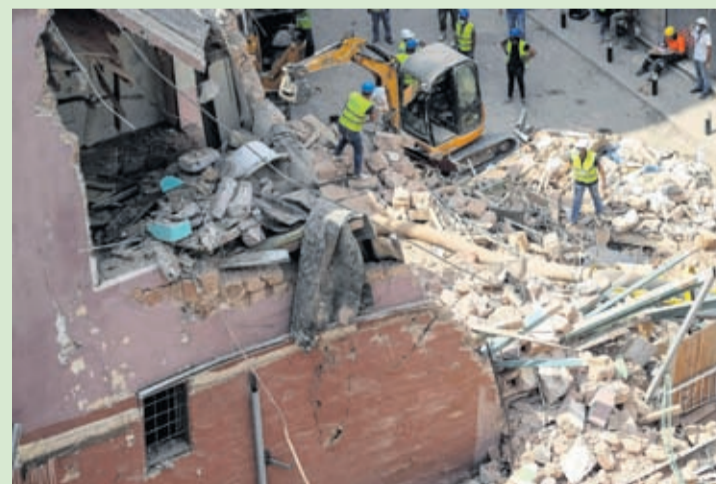
Rescuers search at the site of a collapsed building after getting signals there may be a survivor under the rubble, in Beirut, Lebanon, Saturday, Sept. 5, 2020.
